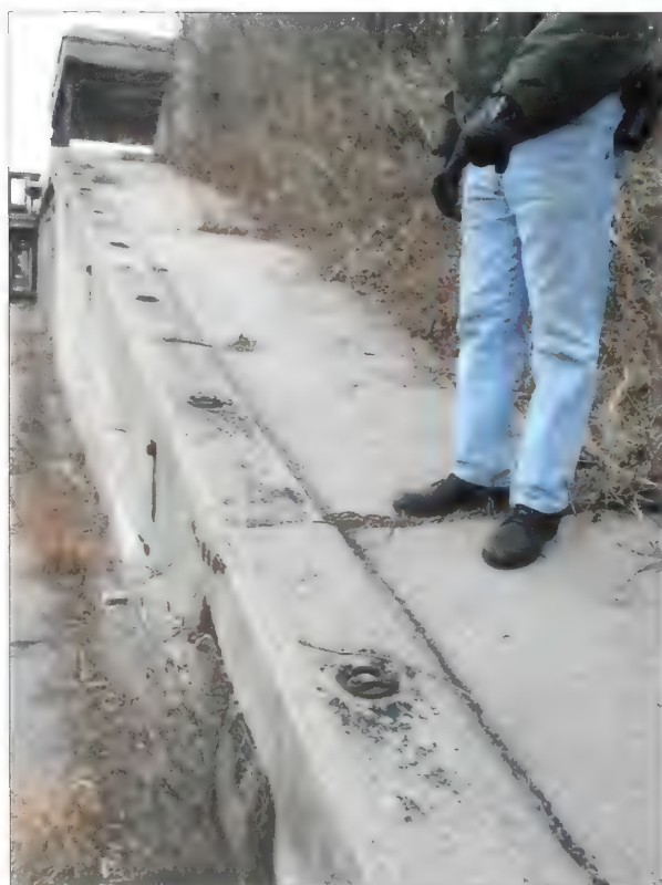
Figure 3.20. View looking northwest at the concrete ramp to gun platform #1, Nine Gun Battery. At transitions between the ground level and gun platforms and also the gun platforms and terreplein, there are stairs and ramps that lack any kind of railing. This ramp has escutcheon plates but lacks a guardrail (Olmsted Center, January 2009).
